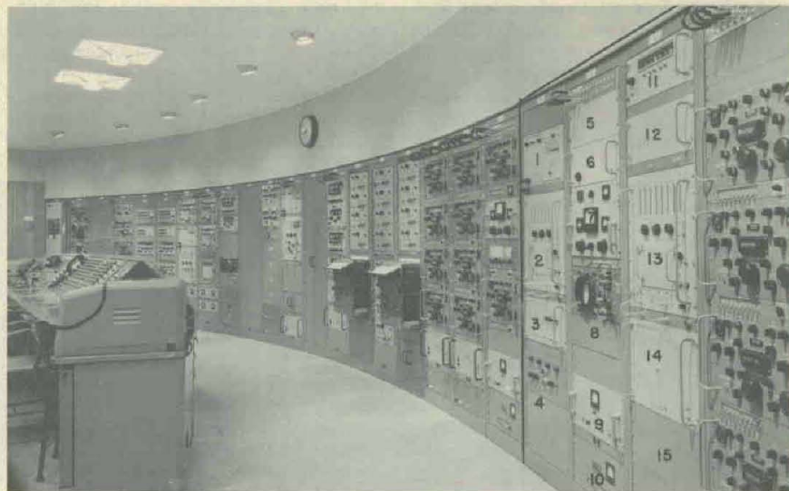
Electronic gear at U.S. Army Signal R&D Lab Astro Observation Center.
